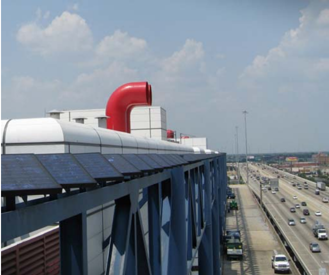
Some of the panels on the U.S. 59 side of the GRB. (Courtesy of Standard Renewable Energy)
